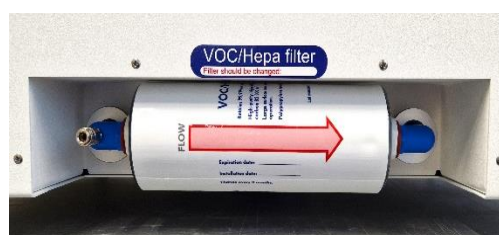
Figure 12.3 Filtre VOC/HEPA correctement installé
